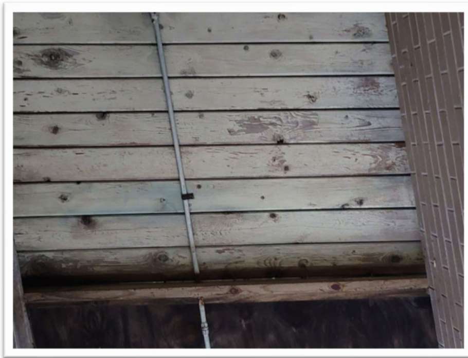
Figure 2.18 - Rotted roof joist.
