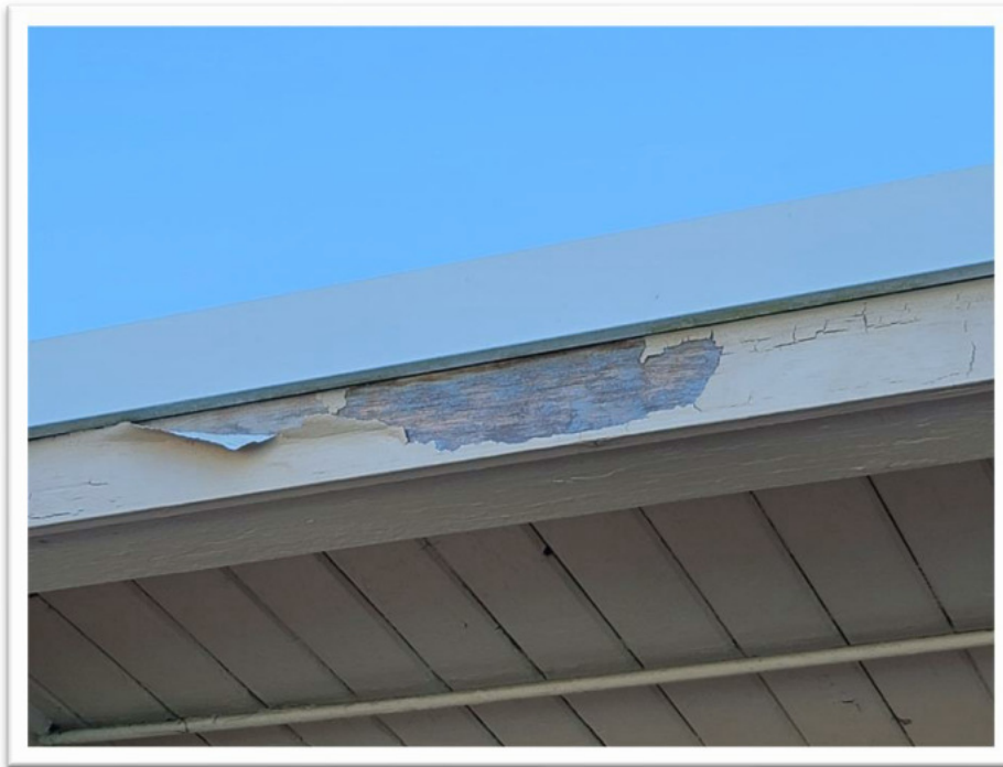
Figure 3.42 - Peeled painting to the fascia beam.
