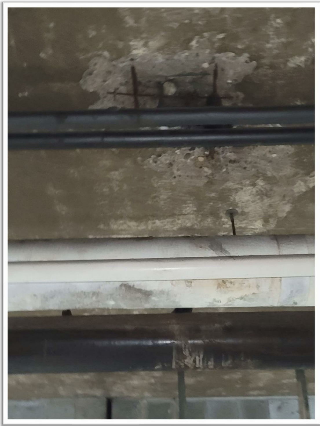
Figure 1.24 - Exposed corroded reinforcement of the ceiling slab.
