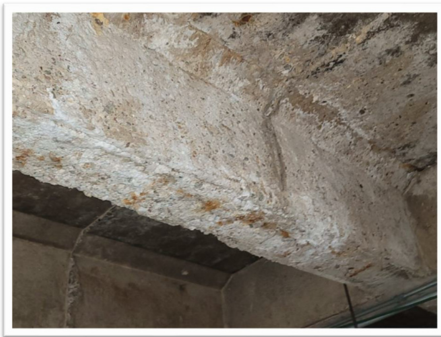
Figure 1.15 - Crumbling and spalling concrete surface.
