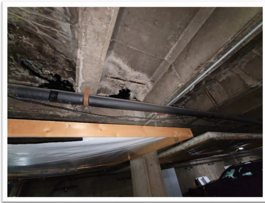
Figure 1.27 - Exposed corroded reinforcement of the ceiling slab with signs of old leakage.
