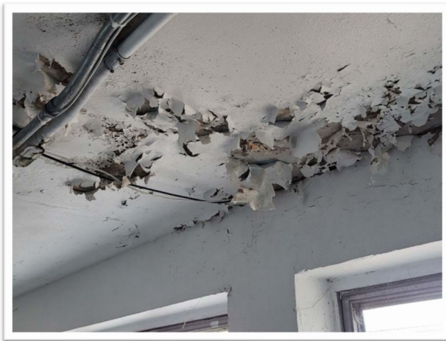
Figure 3.8 - Peeled painting due to severe moisture damage from leakage.
