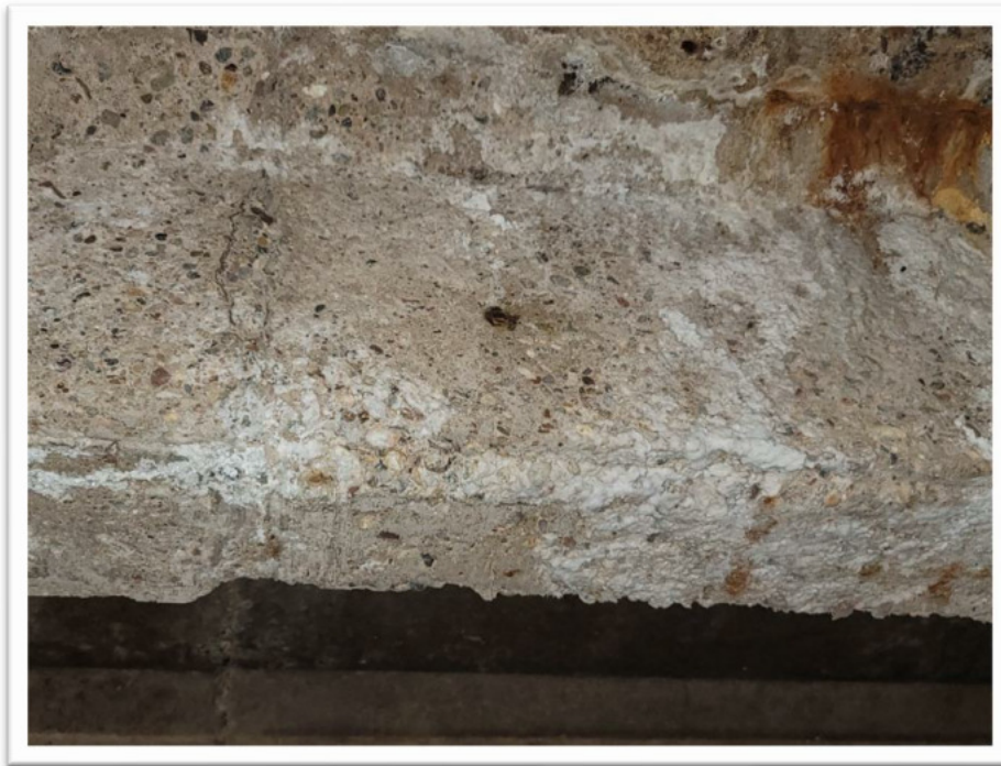
Figure 1.14 - Crumbling and spalling concrete surface.
