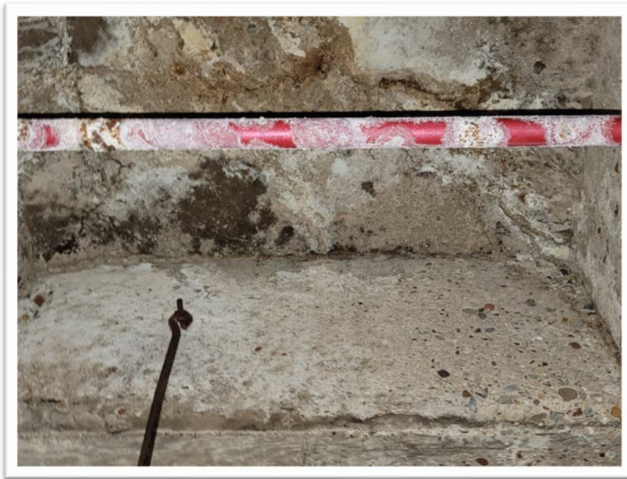
Figure 1.4 - Signs of an old water leakage.
