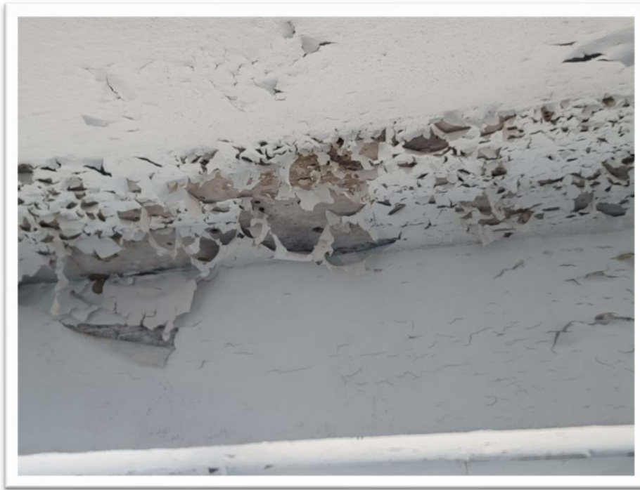
Figure 3.9 - Peeled painting due to severe moisture damage from leakage.
