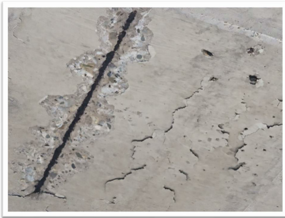
Figure 2.7 - Spalling and crumbling concrete surface through the ceiling slab and corroded reinforcement.
