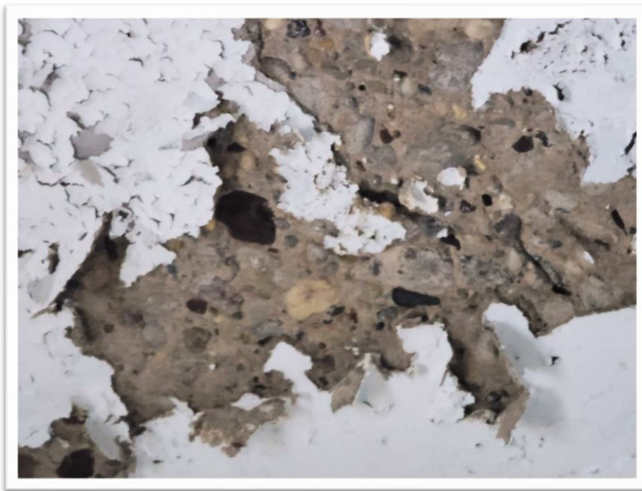
Figure 3.16 - Peeled painting and exposed concrete surface.
