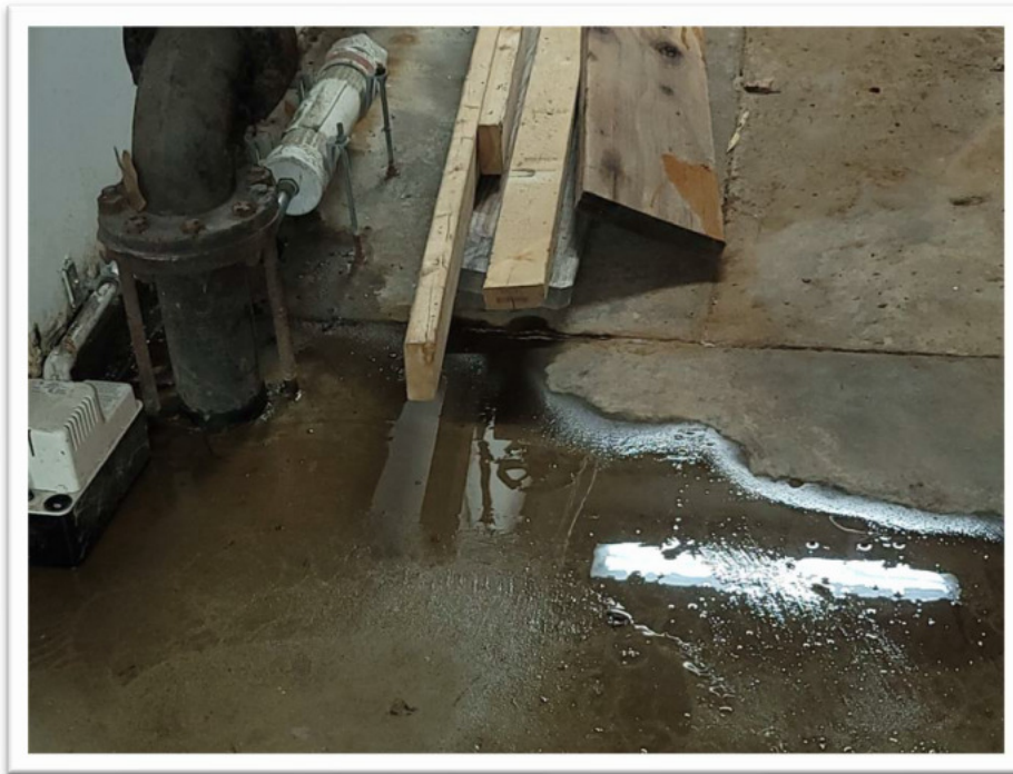
Figure 1.29 - Leakage from the boiler room.
