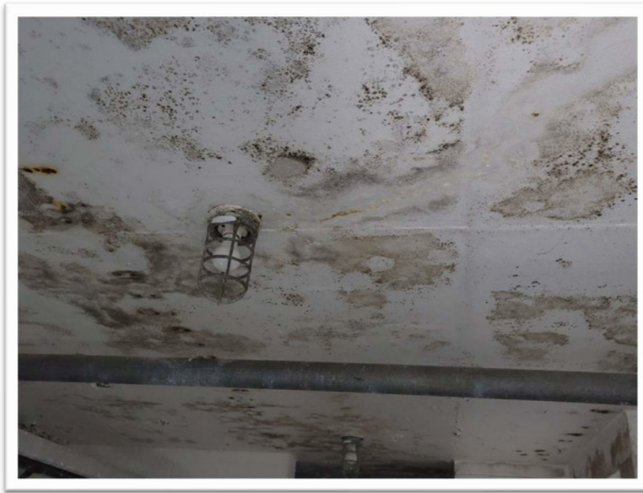
Figure 3.28 - Mold and Severe peeled painting through the ceiling from moisture damage.
