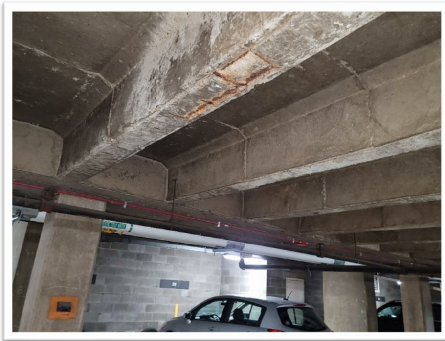
Figure 1.20 - Exposed corroded reinforcement of the beam girder.
