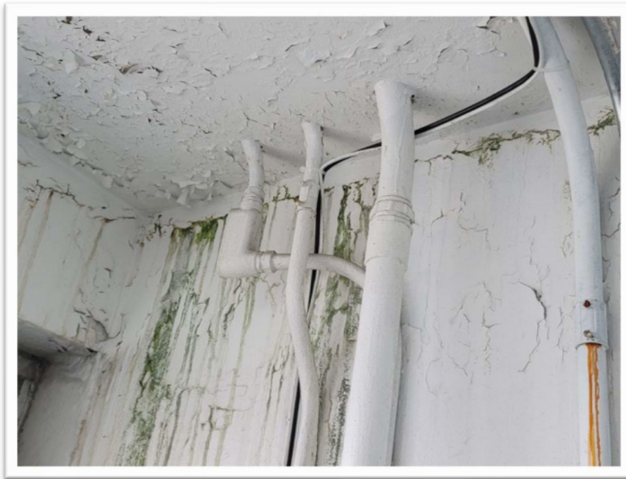
Figure 3.4 - Peeled painting due to severe moisture damage from leakage.
