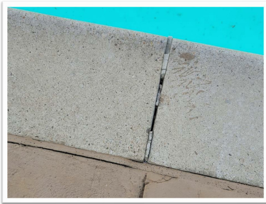
Figure 4.10 - Poor Sealant around the coping.
