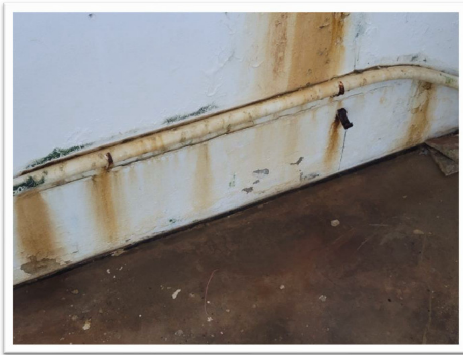
Figure 3.2 - Changing Rooms - Water stains due to severe leakage.
