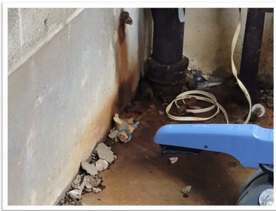
Figure 2.10 - Severe leakage through and around the mechanical system and pipes.
