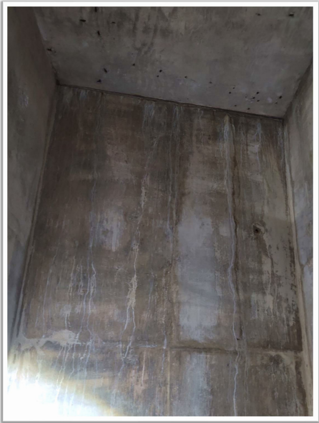
Figure 2.13 - Signs of old leakage through the mechanical room walls.
