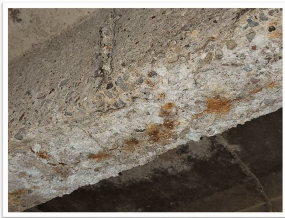
Figure 1.17 - Exposed corroded reinforcement of the beam girder and crumbling surface.
