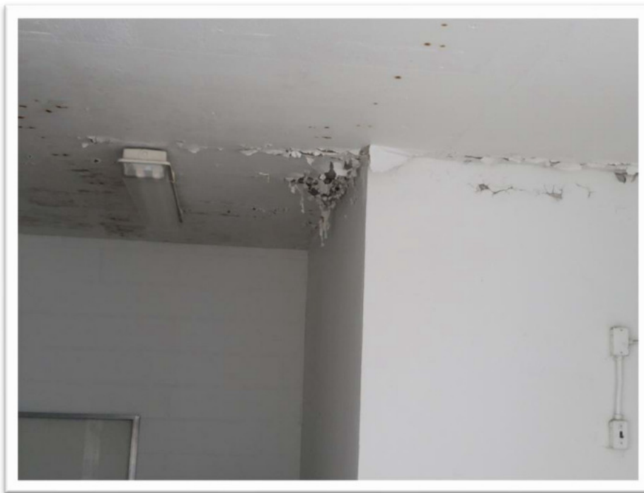
Figure 3.29 - Peeled painting through the ceiling from moisture damage.
