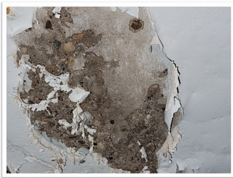
Figure 3.34 - Exposed and spalling concrete surface due to moisture damage.
