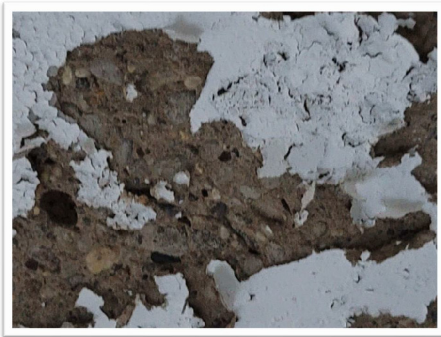
Figure 3.24 - Exposed concrete surface due to moisture damage.
