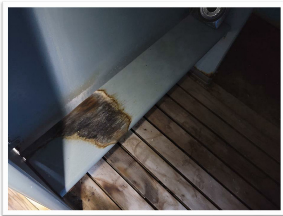
Figure 3.17 - Moisture and Rot Damage.
