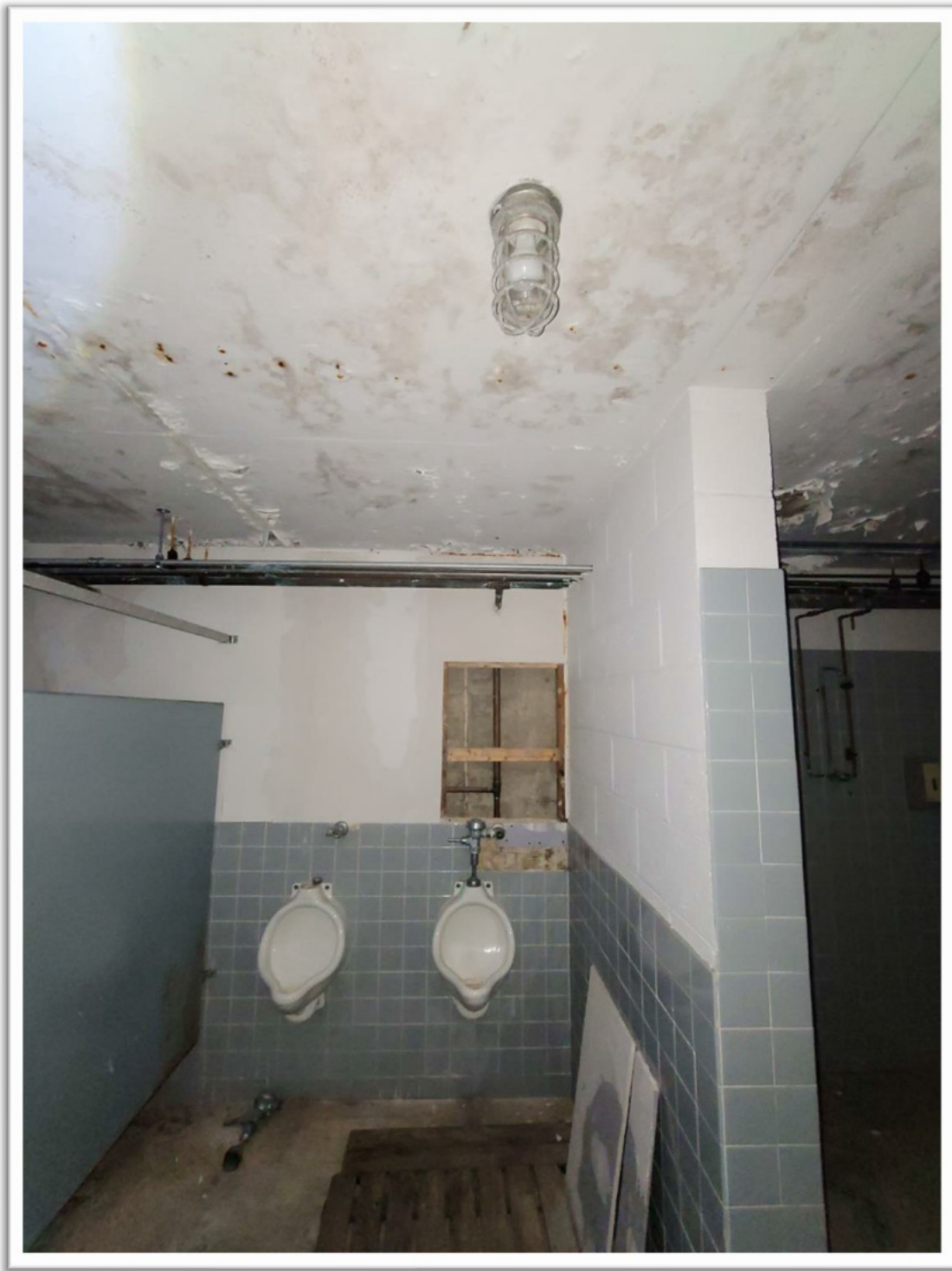
Figure 3.32 - Mold through the ceiling due to high moisture content.
