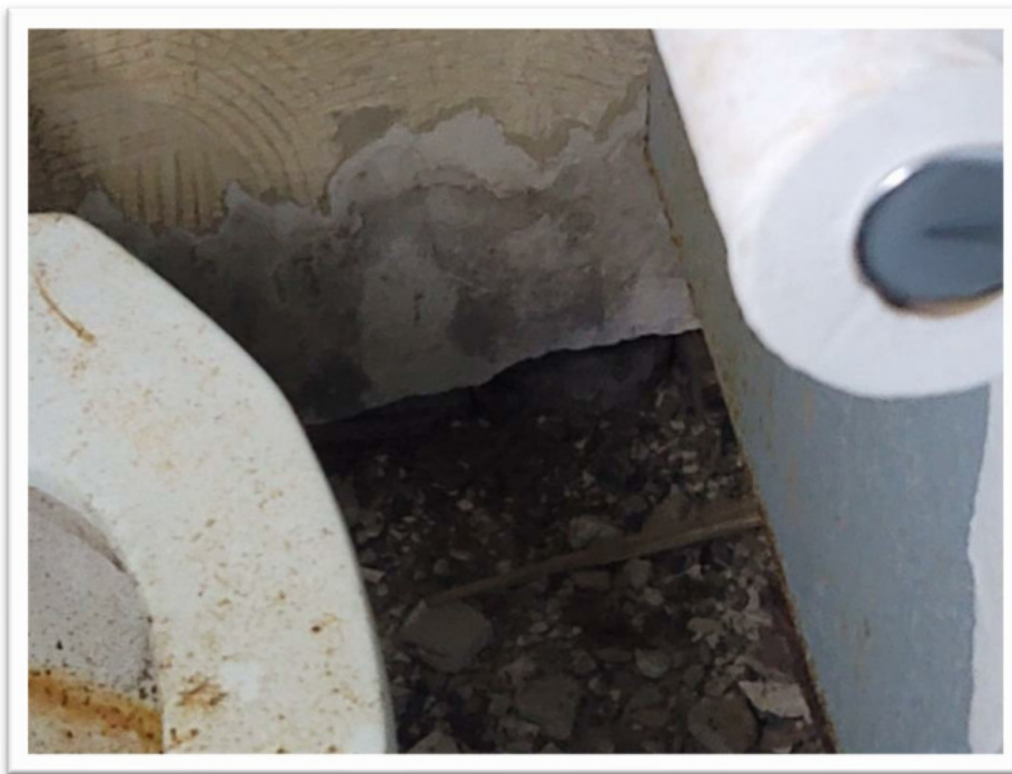
Figure 3.20 - Damage to the floor slab.
