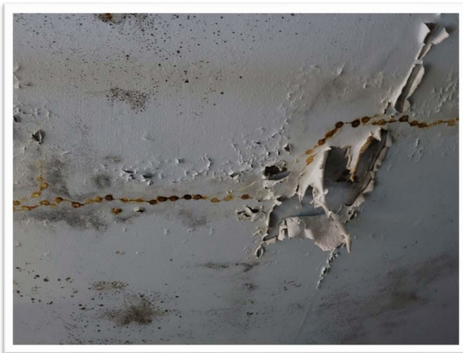
Figure 3.14 - Moisture damage, peeled painting and mold.
