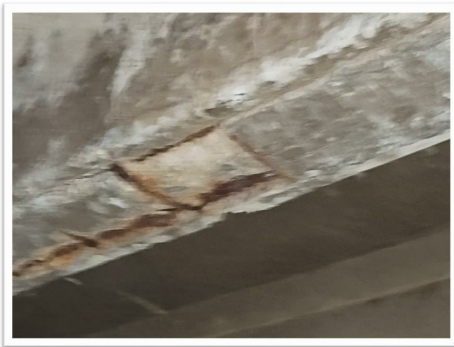
Figure 1.21 - Exposed corroded reinforcement of the beam girder.
