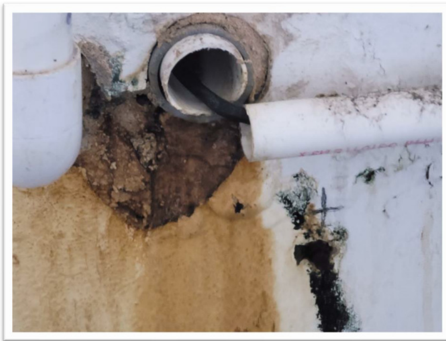
Figure 3.3 - Severe leakage damage.
