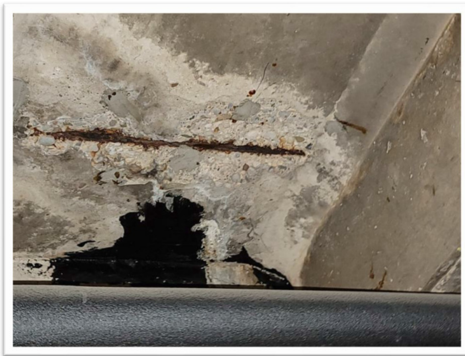
Figure 1.28 - Exposed corroded reinforcement of the ceiling slab.
