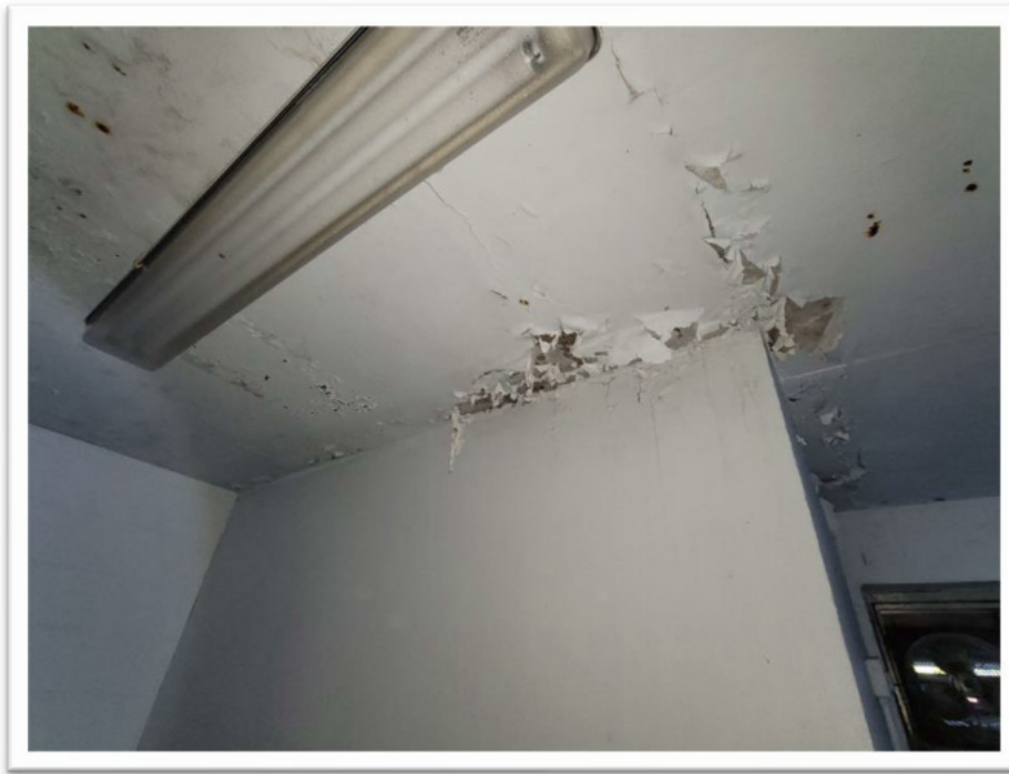
Figure 3.35 - Peeled painting through the ceiling from moisture damage.
