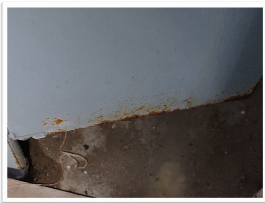
Figure 3.18 - Soft concrete and easily punched slab.
