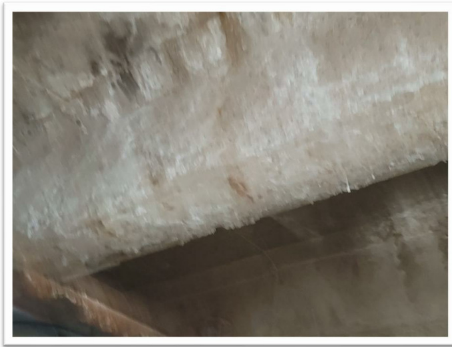
Figure 1.12 - Signs of old leakage with efflorescence deposits.
