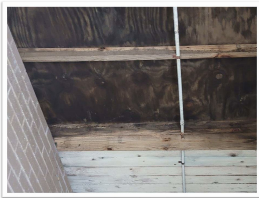
Figure 2.20 - Signs of severe leakage and rot to the roof plywood cover.
