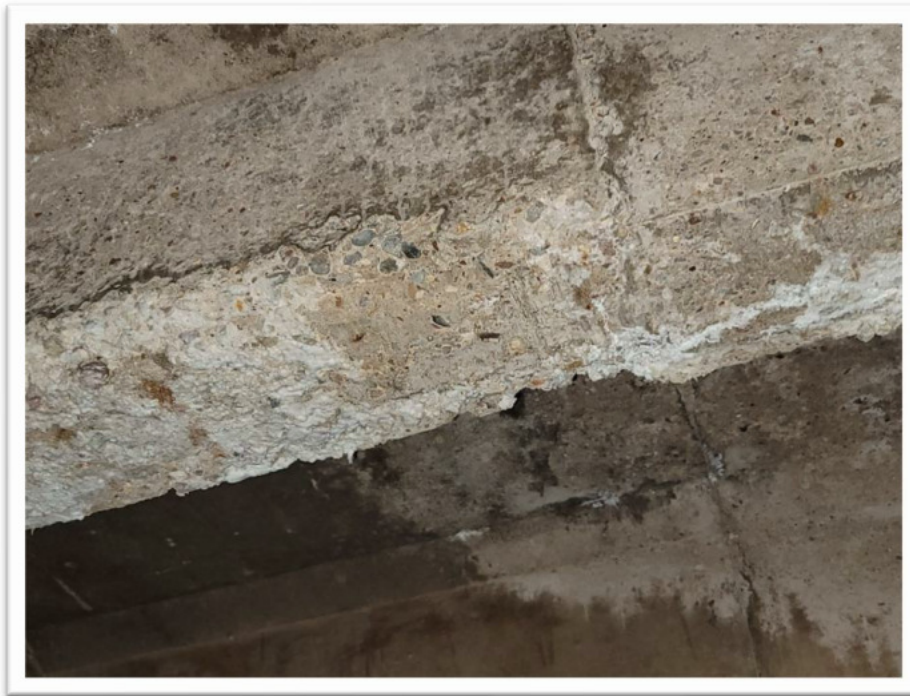
Figure 1.16 - Crumbling and spalling concrete surface.
