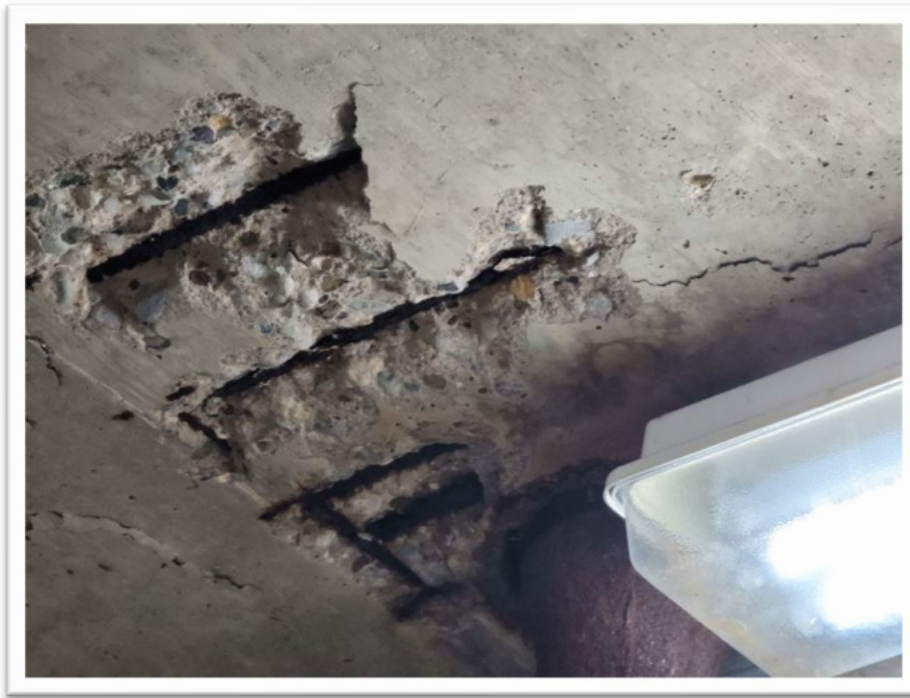
Figure 2.5 - Spalling and crumbling concrete surface through the ceiling slab and severely corroded reinforcement.
