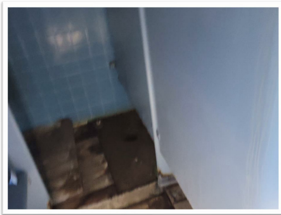
Figure 3.13 - Water damage to the floors.
