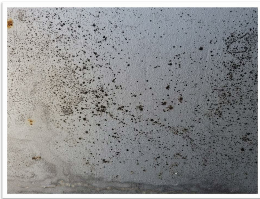
Figure 3.12 - Moisture damage and mold.
