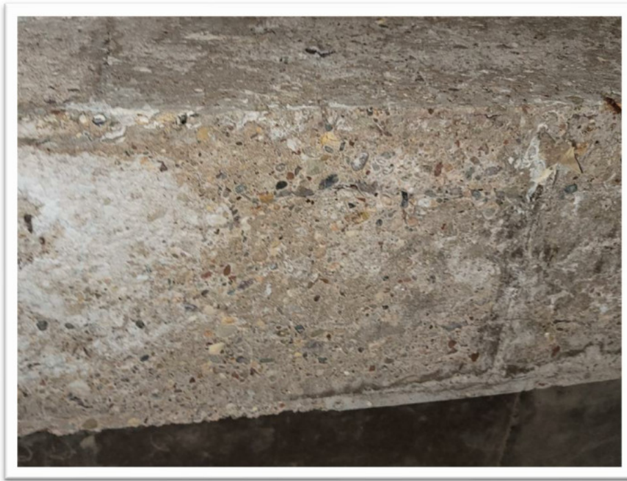
Figure 1.10 - Limited spalling surface that can lead to reinforcement corrosion.
