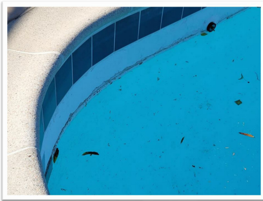
Figure 4.8 - Poor waterline tiles and peeled pool walls.
