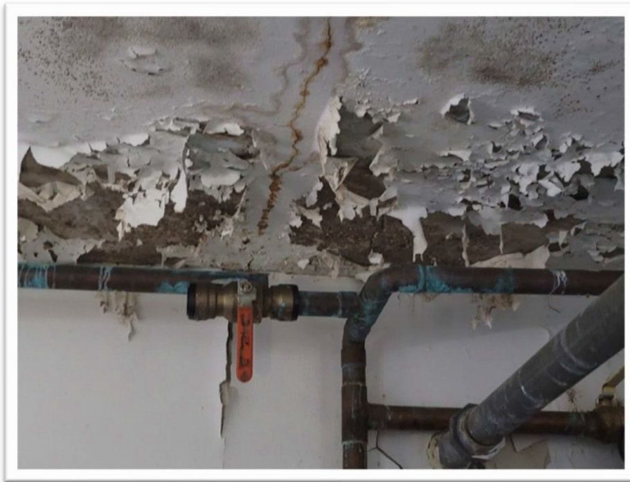
Figure 3.19 - Peeled painting and exposed concrete surface.
