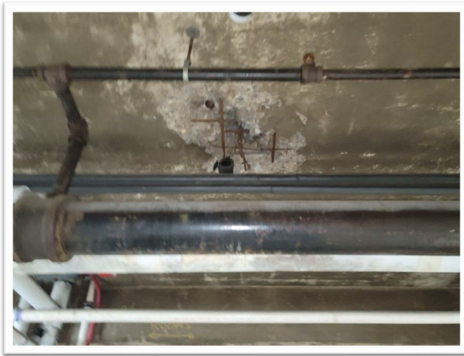
Figure 1.22 - Exposed corroded reinforcement of the ceiling slab.
