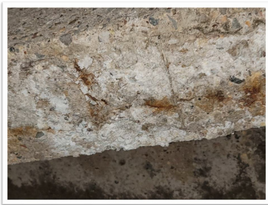
Figure 1.19 - Exposed corroded reinforcement of the beam girder and crumbling surface.
