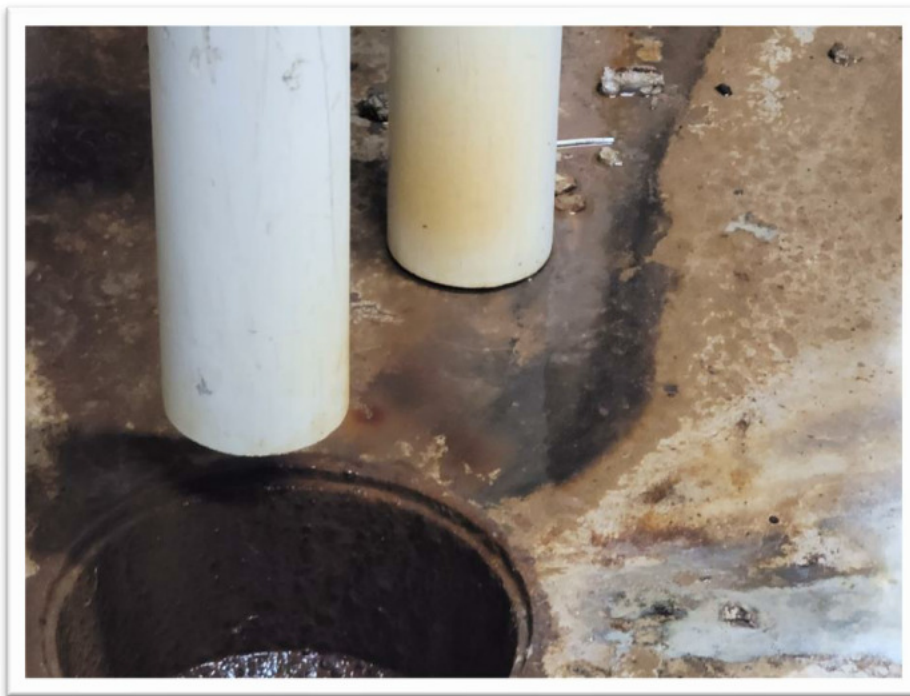
Figure 2.12 - Severe leakage through and around the mechanical system and pipes.
