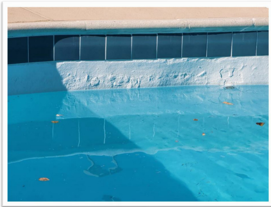
Figure 4.6 - Poor waterline tiles and peeled pool walls.
