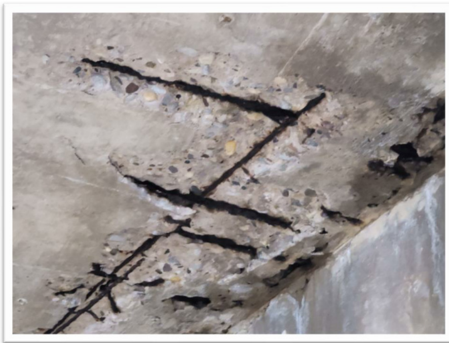
Figure 2.4 - Spalling and crumbling concrete surface through the ceiling slab and severely corroded reinforcement.
