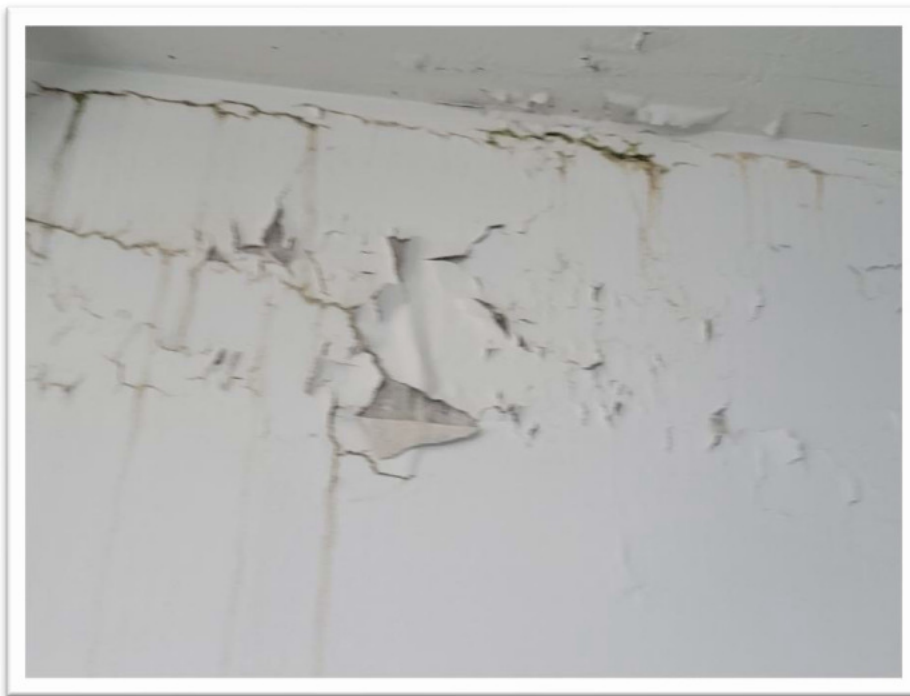
Figure 3.5 - Peeled painting due to severe moisture damage from leakage.
