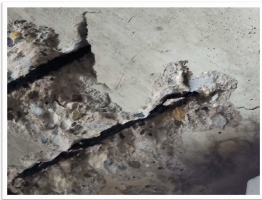
Figure 2.6 - Spalling and crumbling concrete surface through the ceiling slab and severely corroded reinforcement.
