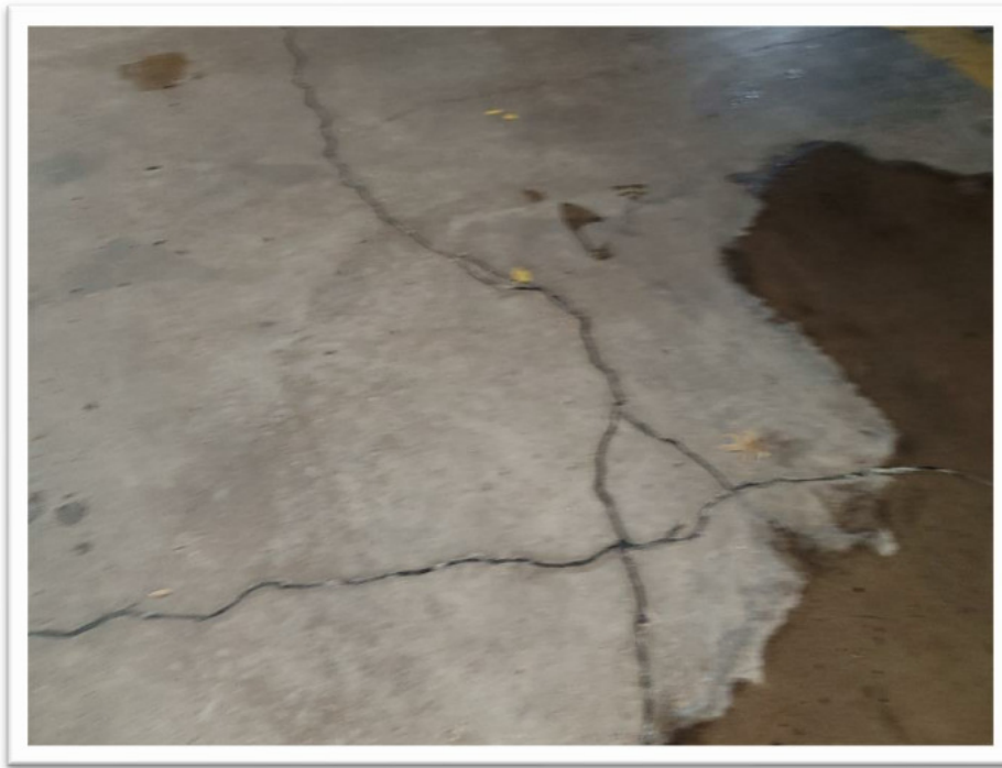
Figure 1.33 - Garage slab settlement cracks.
