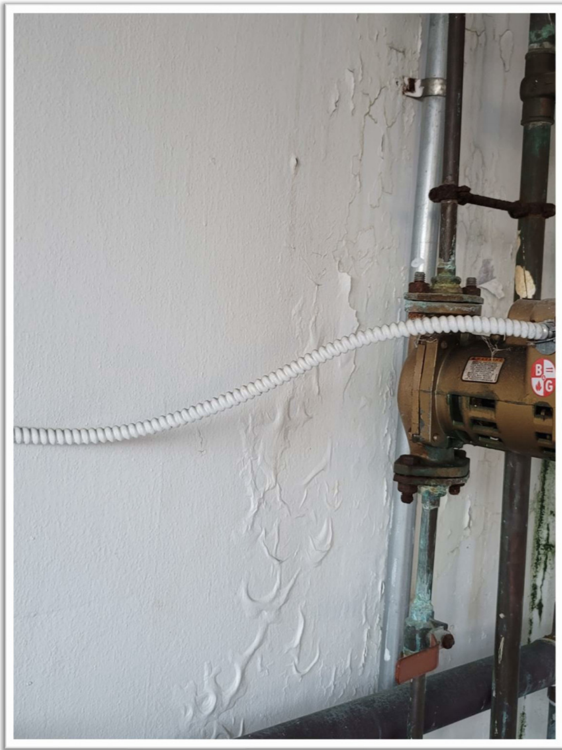
Figure 3.6 - Peeled painting due to severe moisture damage from leakage.
