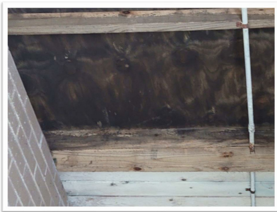
Figure 2.21 - Signs of severe leakage and rot to the roof plywood cover.
