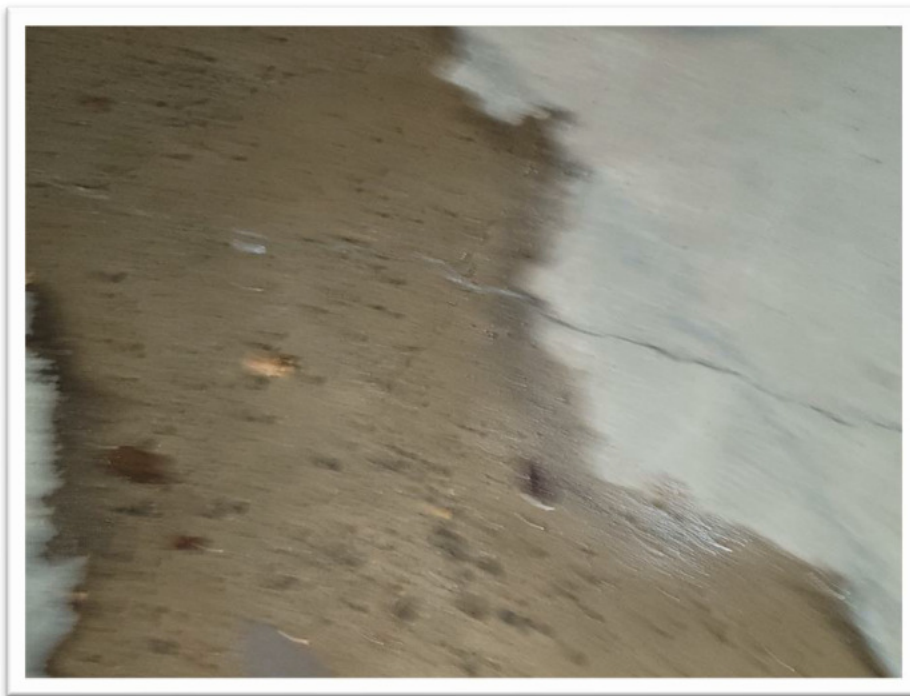
Figure 1.34 - Garage slab settlement cracks.
