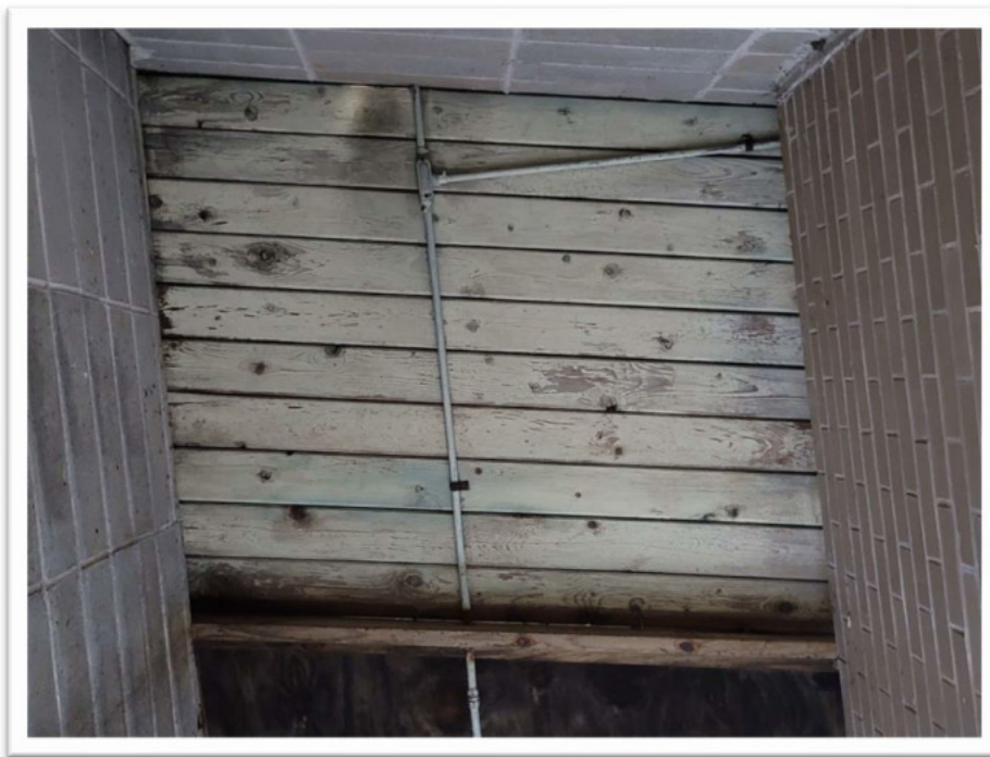
Figure 2.17 - Rotted roof joist.
