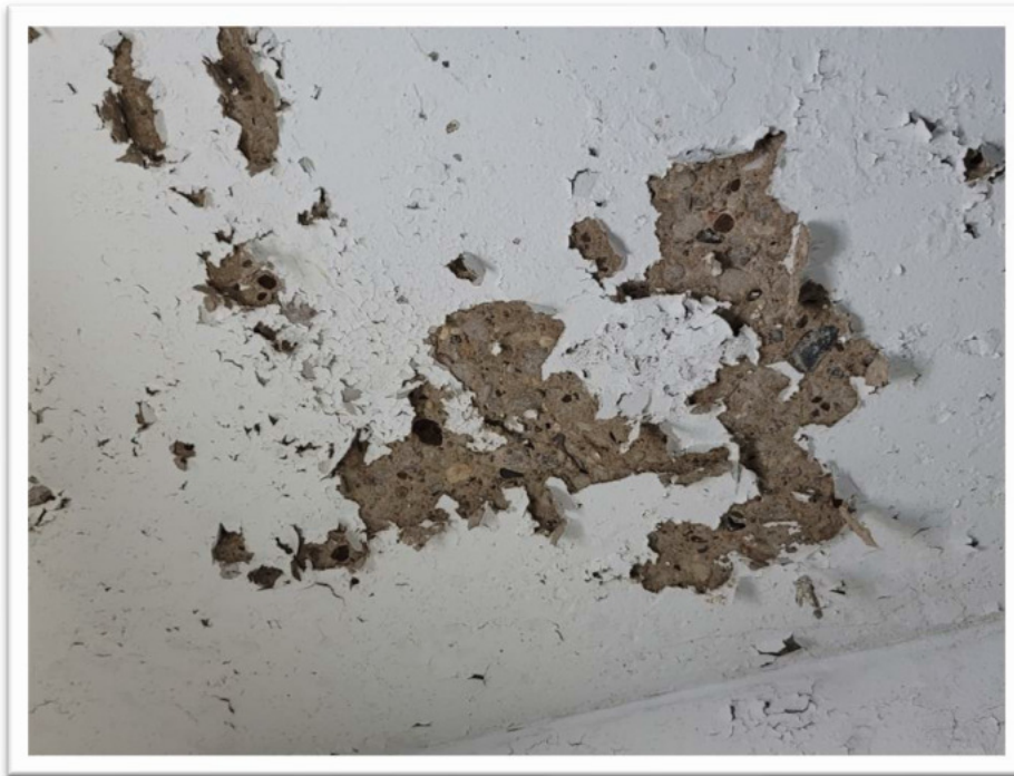
Figure 3.15 - Peeled painting and exposed concrete surface.
