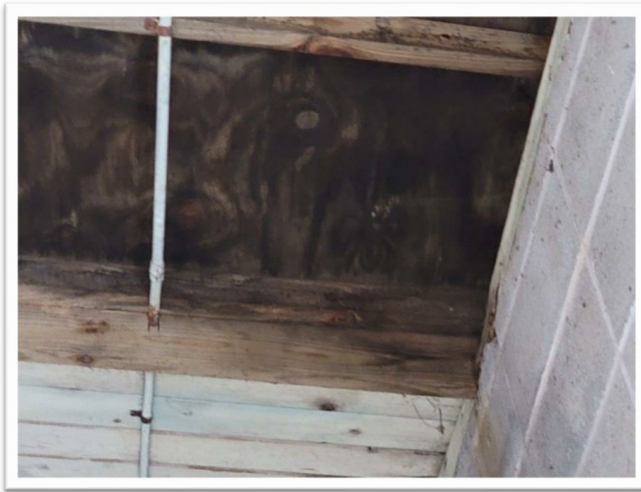
Figure 2.22 - Signs of severe leakage and rot to the roof plywood cover.
