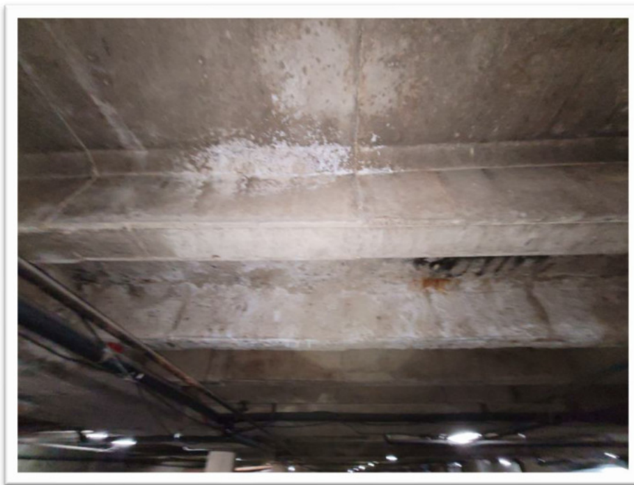
Figure 1.13 - Signs of old leakage with efflorescence deposits.
