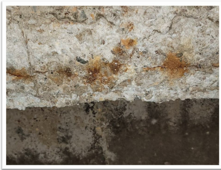
Figure 1.18 - Exposed corroded reinforcement of the beam girder and crumbling surface.
