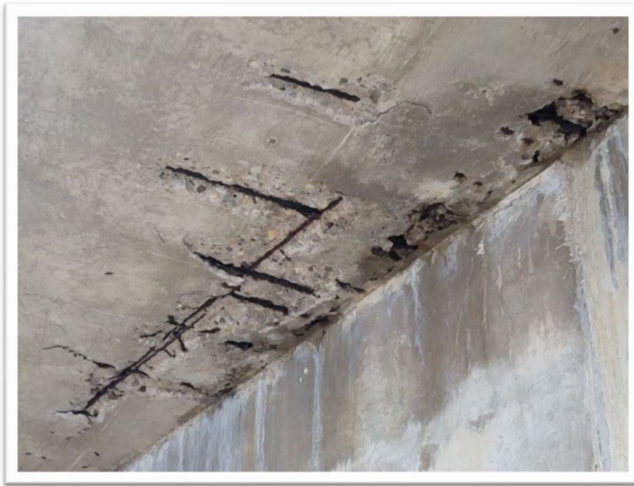
Figure 2.3 - Spalling and crumbling concrete surface through the ceiling slab and severely corroded reinforcement.
