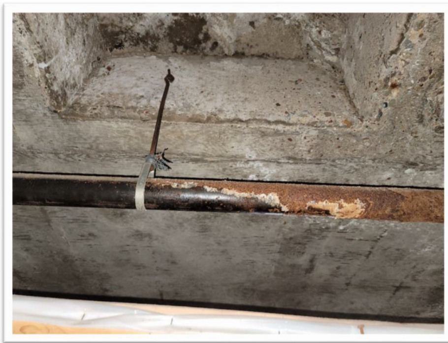
Figure 1.3 - Rusted fire sprinkler pipes.
