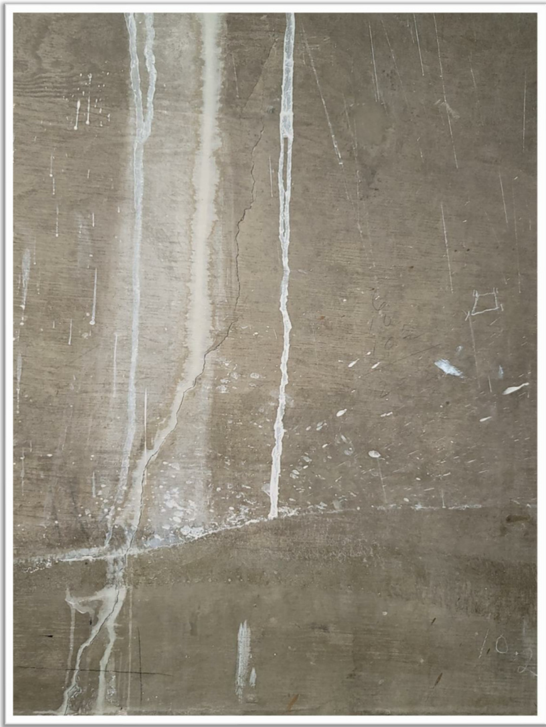
Figure 1.32 - Concrete wall mechanical cracks.
