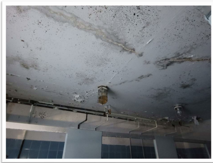
Figure 3.11 - Moisture damage and mold.
