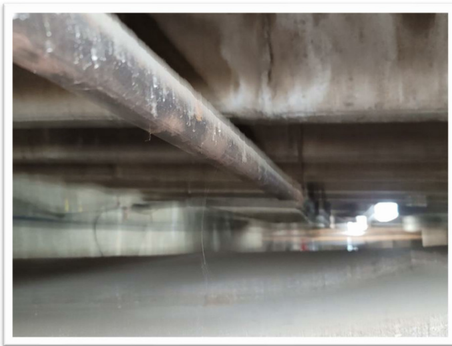
Figure 1.9 - Rusted fire sprinkler pipe.
