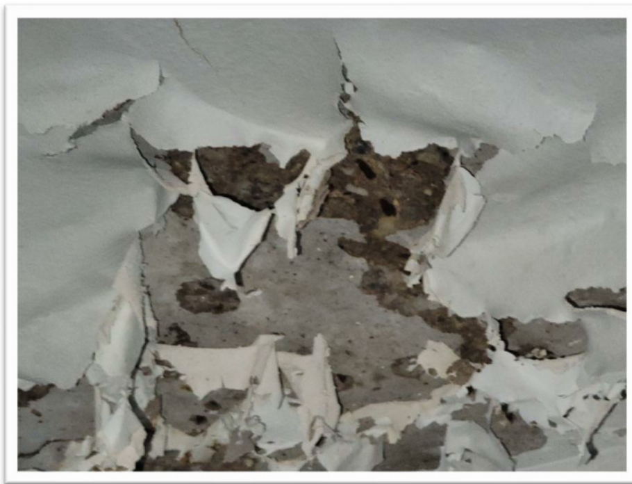
Figure 3.36 - Exposed and spalling concrete surface due to moisture damage.
