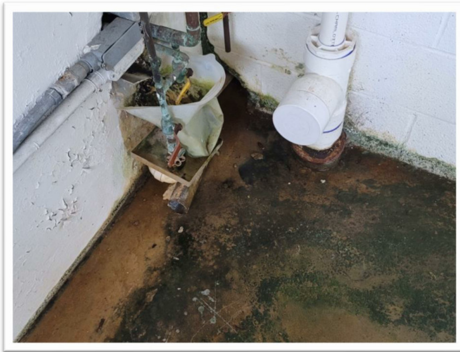
Figure 3.7 - Poor plumbing connections causing water damage to the slab.
