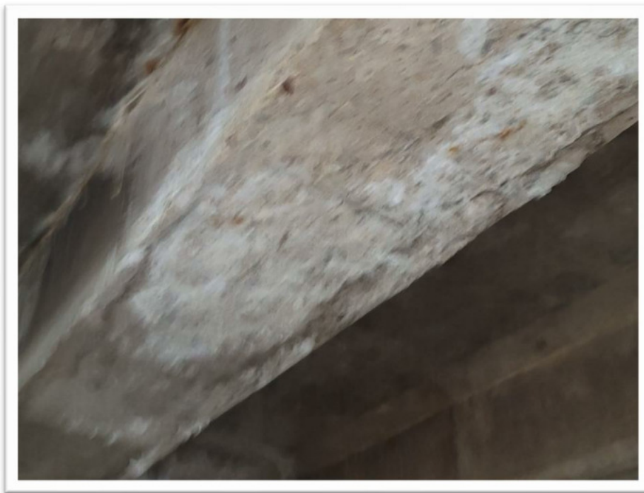
Figure 1.11 - Crumbling and spalling concrete surface with efflorescence deposits.
