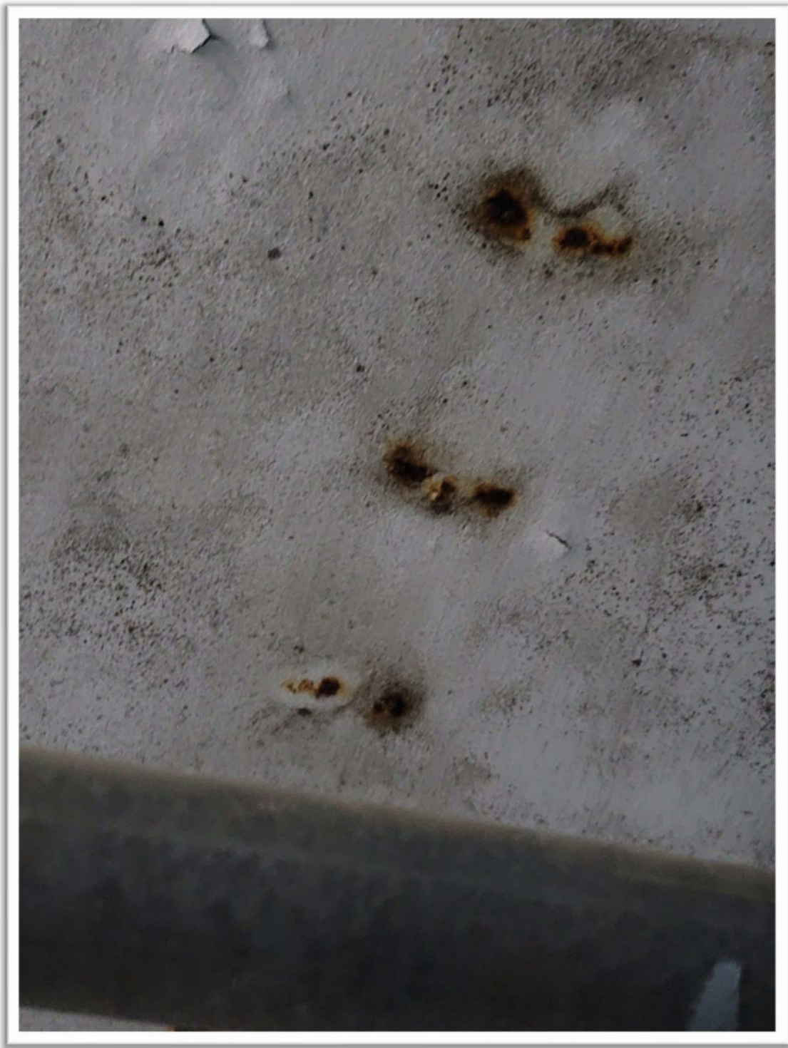
Figure 3.23 - Mold through the ceiling.
