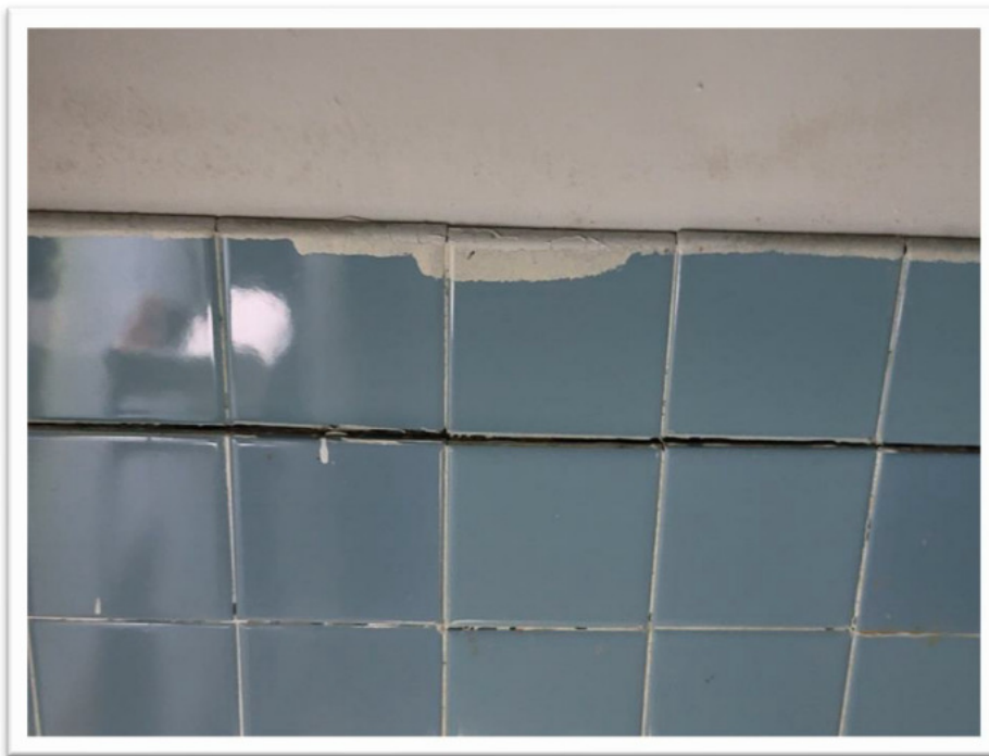
Figure 3.22 - Damage to the tile from the moisture.
