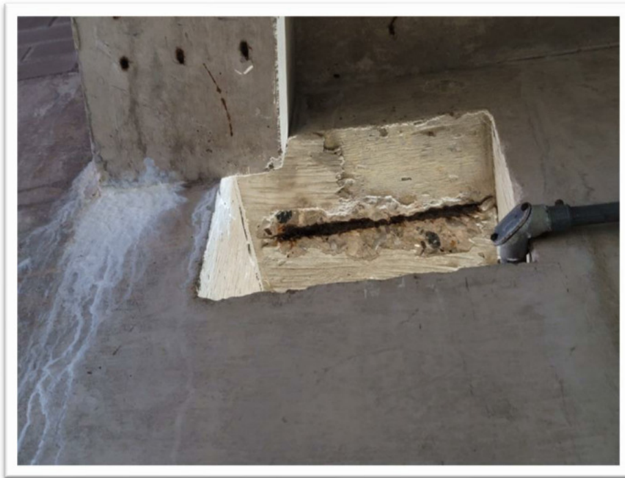
Figure 2.14 - Exposed corroded slab reinforcement.
